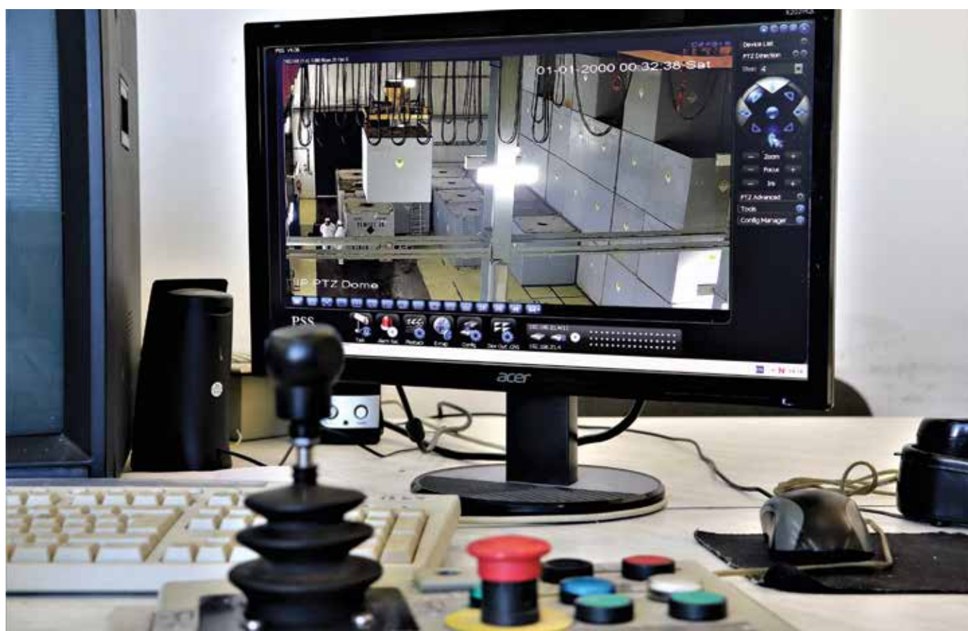
Control room in Specialised Division RAW, Photo SE RAW
