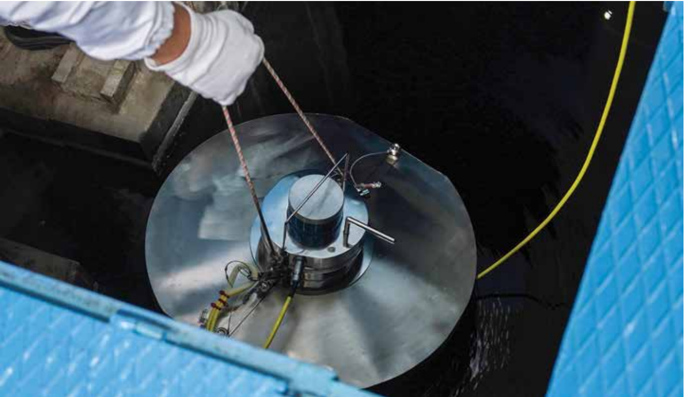
Spent Fuel Storage Facility, Photo Kozloduy NPP
