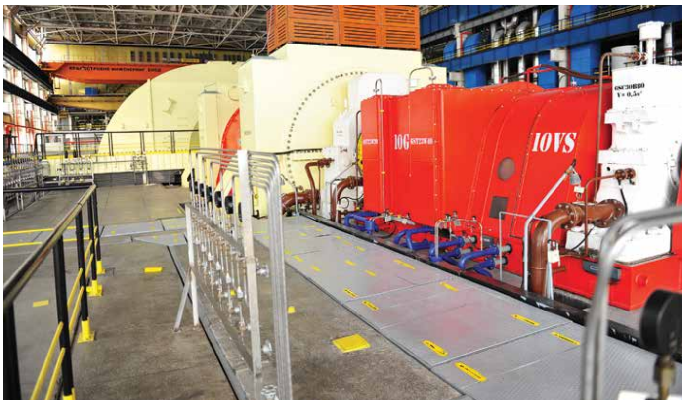
Turbine Hall of Unit 6, Photo Kozloduy NPP
