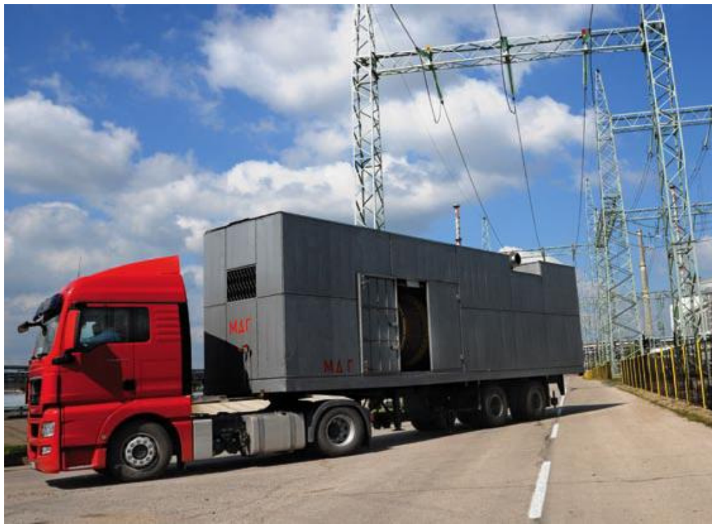
Figure 6.1-3: Kozloduy NPP. Mobile diesel generator.
